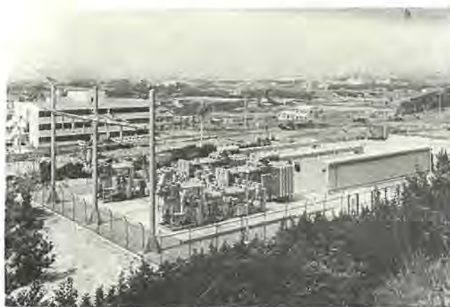
図4. 名古屋市水道局 猪高配水場納め77 kV GIS 77 kV GIS for Idaka water supply plant of the Nagoya city water works bureau.
