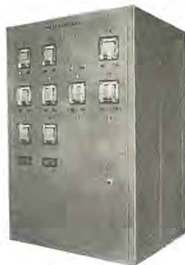
図 5.6(b) 傍受局計器盤 (谷ヶ原) Fig. 5.6(b) Telemetering panel of substation.
