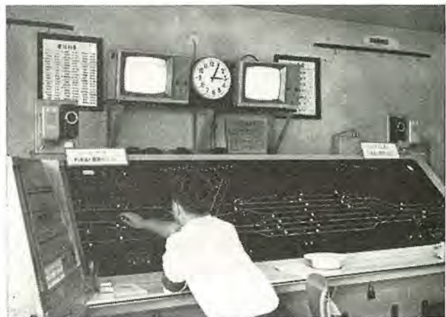
図 11-35 国鉄宮原第一信号扱所 IT V モニタ IT V monitor used at train control room of the Japanese National Railways.
