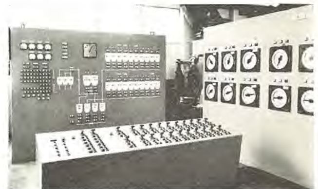
図 4-79 照光盤および操作盤 Illuminated graphic panel and control desk.
