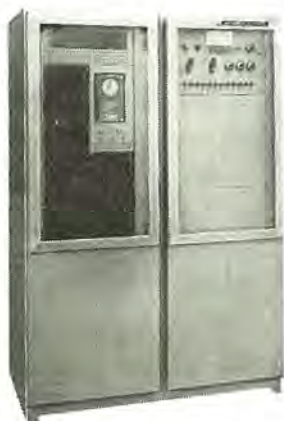
図 12-16 無効電力制御計算機 Computing equipment for reactive power control of power system.
