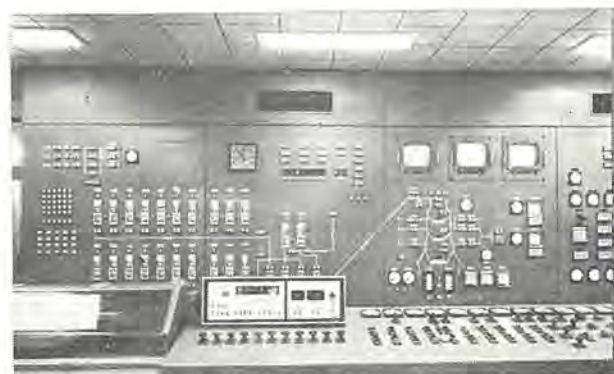
図 4-4 照光盤および操作盤 Illuminated graphic panel and control desk.
