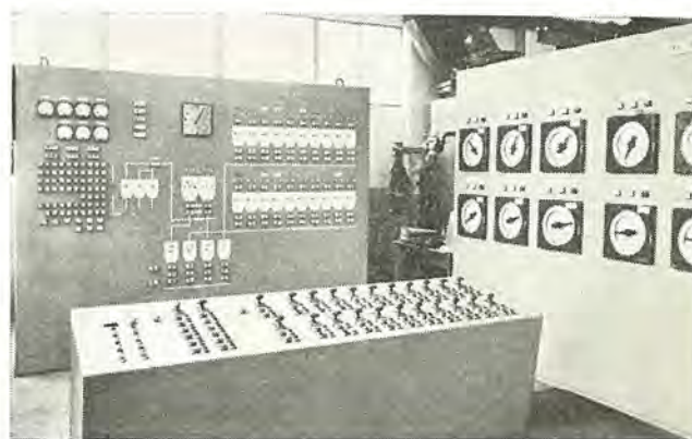
図 4.8 計量管理室運転室 Fig. 4.8 Measuring control and operation room.
