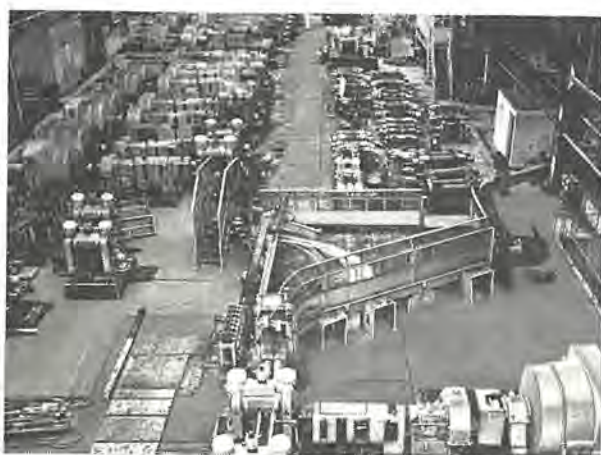
図 2.5 富士製鉄釜石製鉄所線材ミル用電気品 Fig. 2.5 Electrical equipment for wire rod mill at Kamaishi Works, Fuji Iron and Steel Co.
