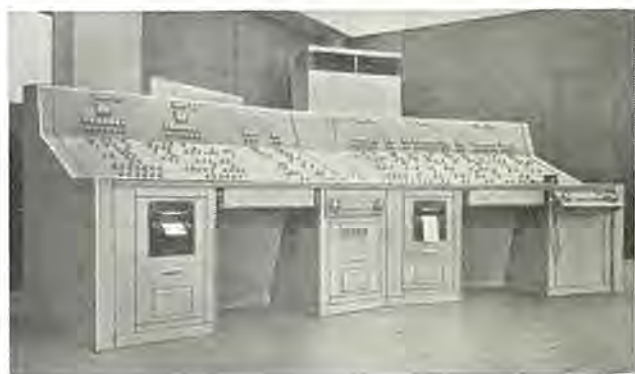
図 1.35 集中制御盤 Fig. 1.35 Centralized remote control equipment
