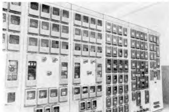
図 5.3 補助盤 (継電器盤) Fig. 5.3 Auxiliary panel (Relay board).
