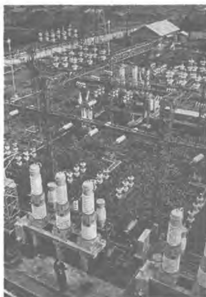
19 図 受電側母線と V.C.B Fig. 19. View of A-C bus structure and Porcelain type oil circuit breakers.
